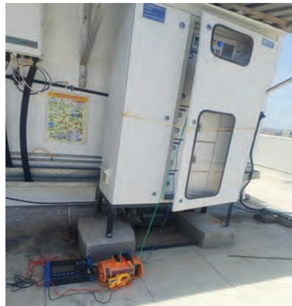
Fig. 4. Solar connected single phase induction motor through power quality analyzer.
